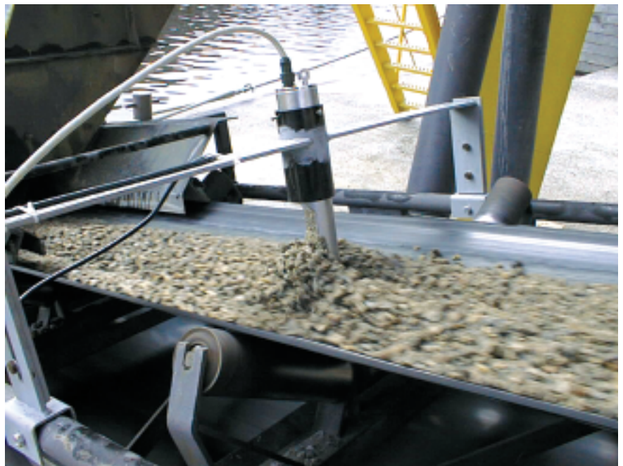
Typical installation of a digital microwave moisture sensor on a conveyor belt
