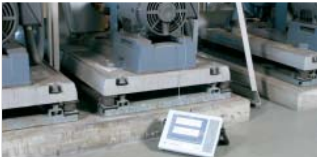
Vibration measurement in a plant using the CF-7200 and an NP Series Accelerometer
